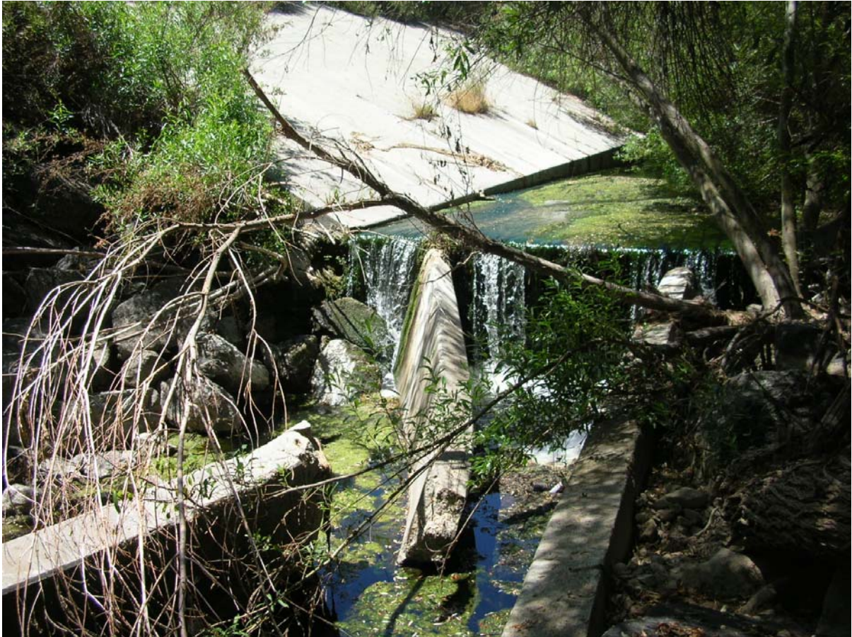
Looking upstream at approximate Station 18+59 □ Failed cut off wall and vertical drop in channel invert.
